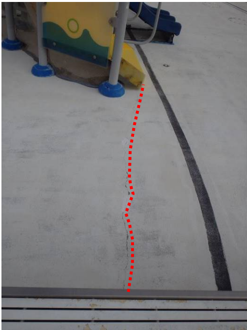
Photograph 7: Crack (red dashed line) in the floor slab of the zero-entry area near the kids' water feature.
