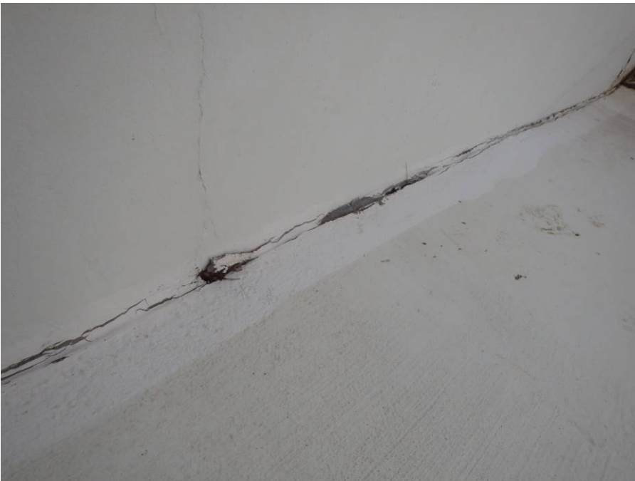
Photograph 5: Distorted slab to wall joint present along the ramp down to the diving area.
