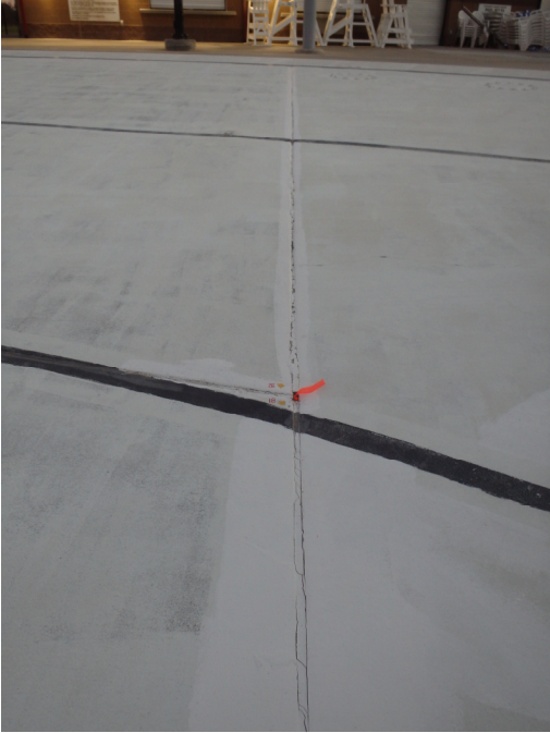
Photograph 4: Slab expansion joint in the zero-entry area that is distorted and found to leak by BAI.
