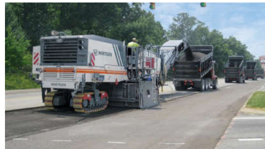
Cold Milling will remove the upper section of the existing street surface.
